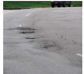
Asphalt mat failure under repeated loading when the subgrade has failed (Above)
