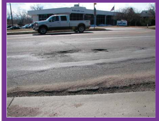
Rutting and Slippage in a city street
