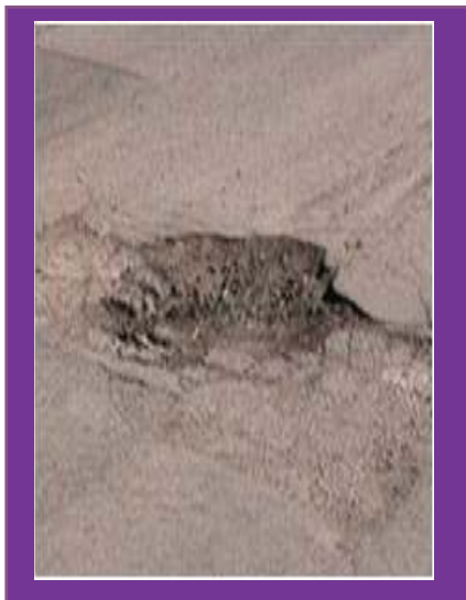
A Pothole forming in a city street
