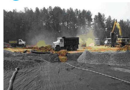
The infiltration bed serves as an underground detention basin
