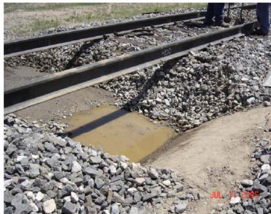
Figure 3. Asphalt Damage and Standing Water
